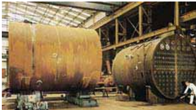
A typical waste heat boiler of the shell and tube pattern under construction. Note that there is no combustion chamber, only tubes.
